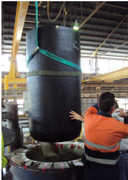
Fig. 3. A cylindrical crucible is installed in an induction furnace.
