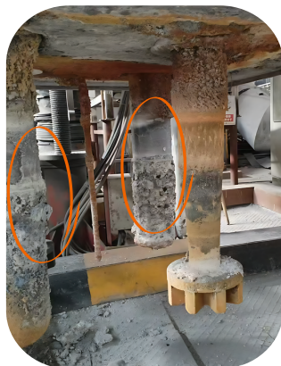
Heavy dross accumulation on Ceramic Heater Sheaths
