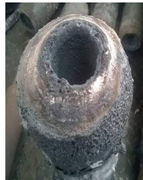
Less erosion observed after 5 days
