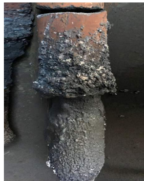
Break after use due to severe erosion
